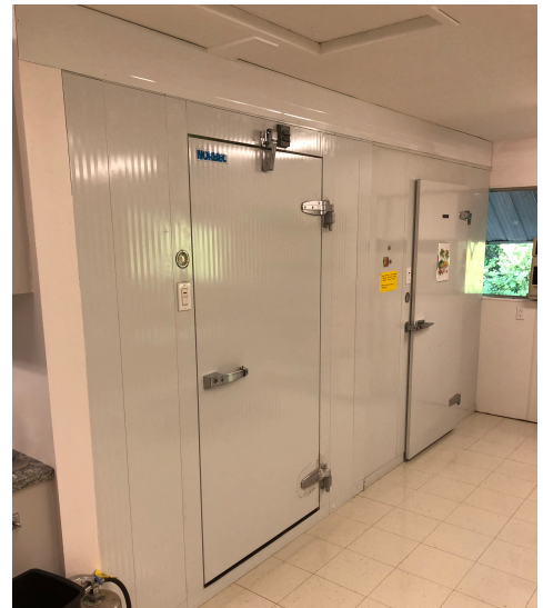
A view of our new walk-in freezer, right beside the older walk-in fridge!
